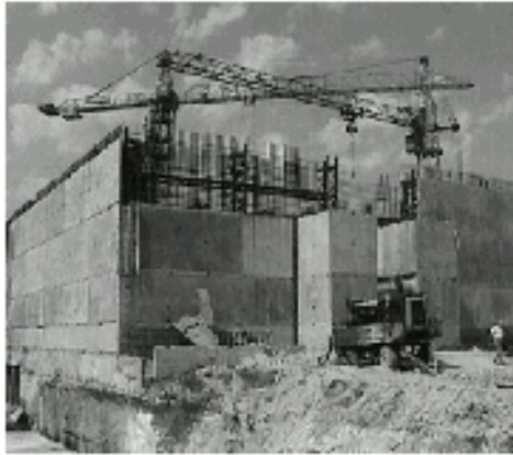
Fissile Material Storage Facility under construction at Mayak, financed by the US Cooperative Threat Reduction program.
