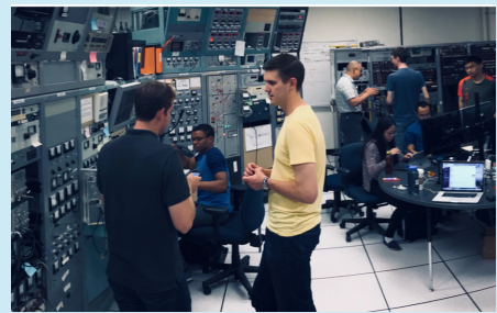
Tandem Control Room at TUNL [S71]
